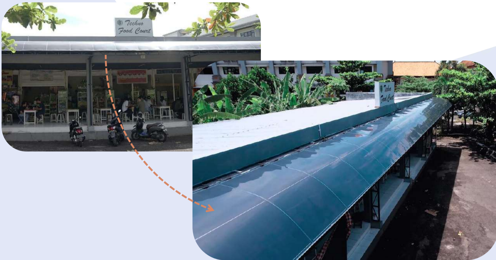
Flexible Solar Panel Installation at the Canteen of Engineering Faculty of Udayana University
